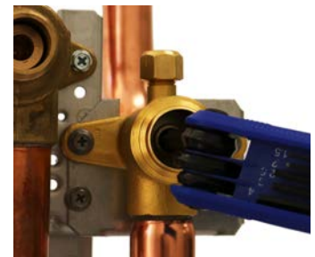
Opening the Service Ports.
